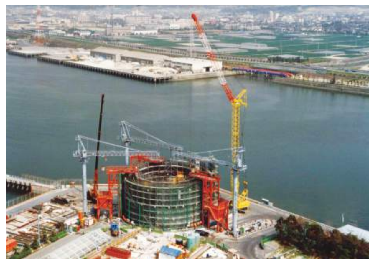
Shin-Nagoya Thermal Power Plant Shaft
